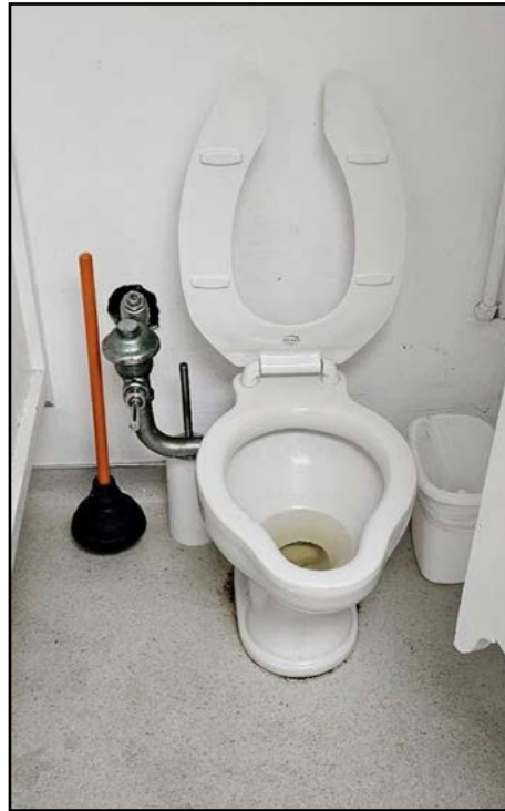
One of the old toilets, which were likely originally installed in the 1950s.
