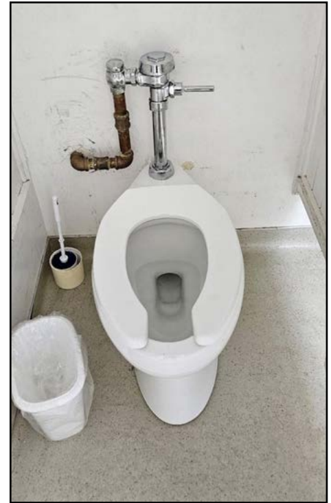
One of the new, more efficient toilets installed last month.
